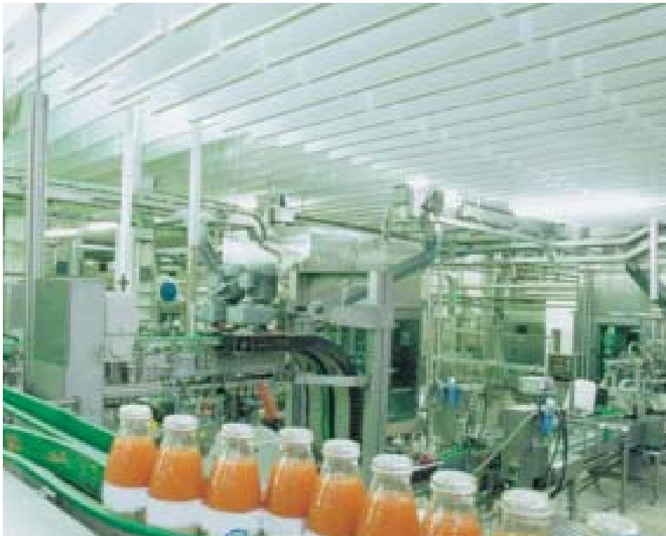
illbruck wetroom absorber, bottling plant, Pfaffenhofen/Ilm, Germany
